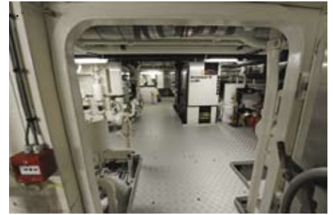
The pump room aboard the ICON 62
